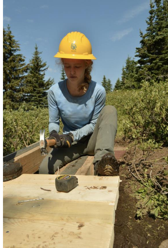
SCA Crew member Rachel Hultman installs decking on a timber bridge at the Heather Trail in E.C. Manning Provincial Park, British Columbia
